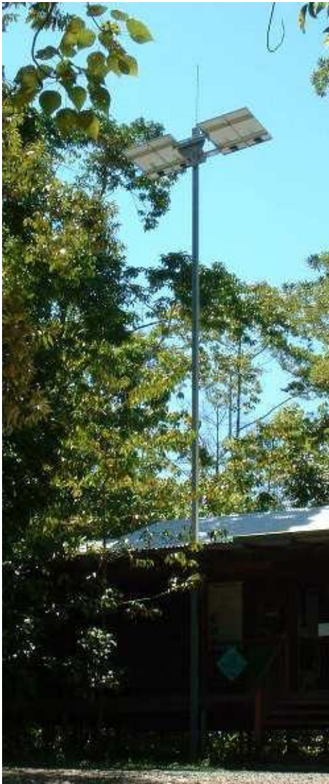
Fig 28 Elevated solar arrays
