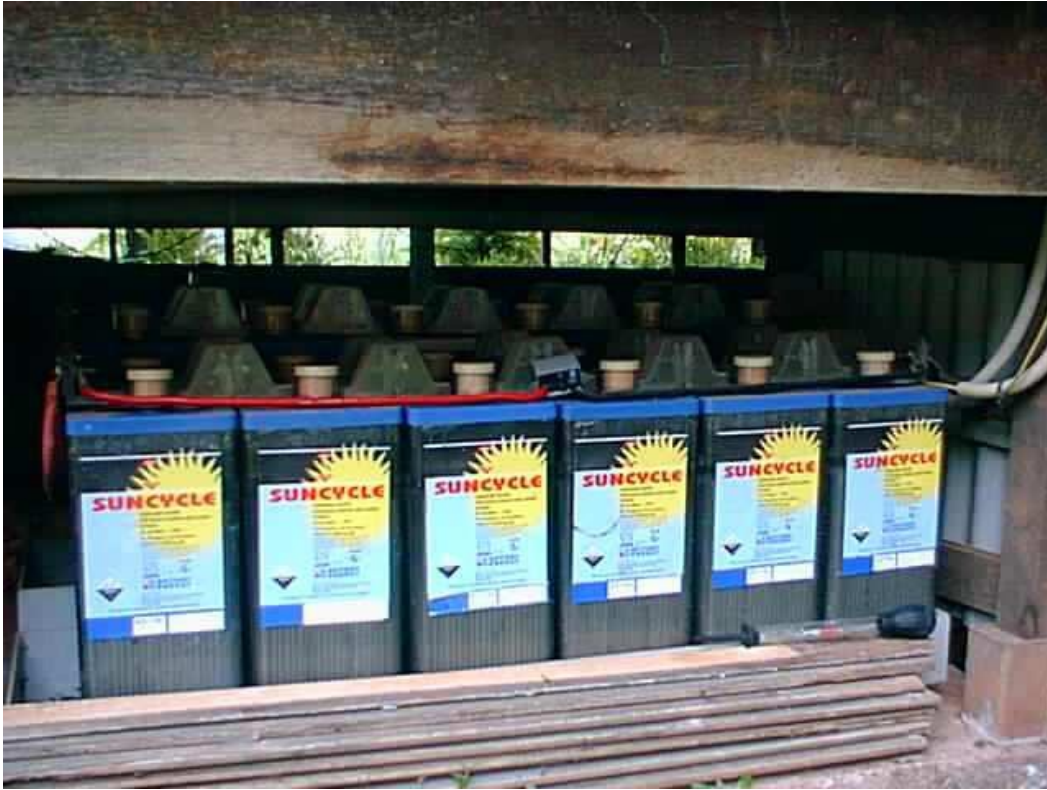
Appendix 2 Fig 4 Battery located under a shed floor. Such locations (quite common in the Daintree) make routine maintenance and cleaning of the battery tops a very daunting task. At least the installer put the batteries in an appropriate plastic catch tray, which also stops organisms moving up and growing up between the battery cases, and the batteries are kept cool and well ventilated (by default). The de- sulphator is obvious on top of the batteries.
